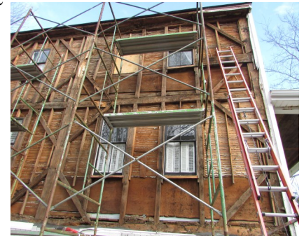
Recent renovations at John Coffin's house at Mast Landing. This view shows the eastern side of the house. The marked edge is on the bottom of the lower wainscoting board, below the window center right.
